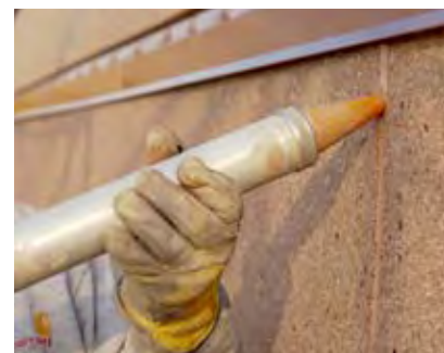
To make sure that nothing would mar the appearance of the sleek and attractive façade over time, Spectrem 4-TS Silicone Sealant formulated with Tremco's patented Advanced Silicone Technology was used to provide a perfect match to the EIFS. Its superior performance enhances the life and durability of the cladding system, protects against dirt pickup and minimizes maintenance.
