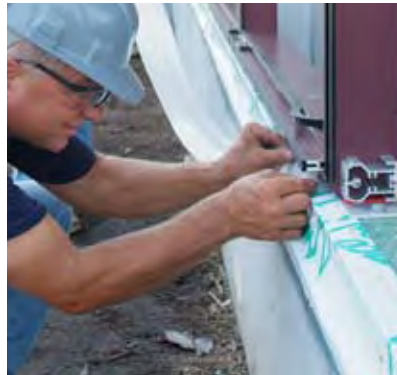
Tremco's proprietary Proglaze® ETA Engineered Transition Assembly System 3 ribbed silicone sheet was plugged into the mullion race at the sill and at the head and sealed in place with Spectrem 1 silicone sealant.
