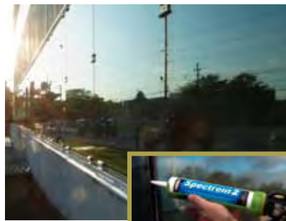
A vertical weather bead of Tremco's Spectrem 2 Silicone Sealant was applied between the glass units, creating the look of a continuous ribbon of glass and a comprehensive, compatible, weathertight façade assembly ready for the installation of the Dryvit Outsulation MD exterior cladding.
