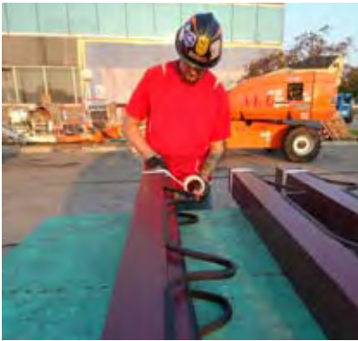
Framing members for the high-performance Kawneer 1600 Wall System arrived at the site with the peroxide EPDM gaskets from Tremco pre-installed.
