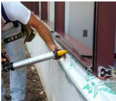
The metal and ExoAir 110 surfaces were cleaned in preparation for the engineered transition assembly which provides a durable and secure seal from the window assembly to the wall assembly. Tremco's Spectrem® 1 Silicone Sealant was applied to the metal race at the sill.
