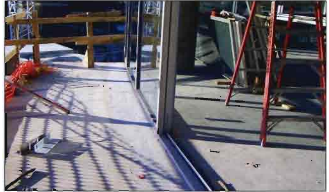
Silicone sealant used at all sill locations, jambs, and head of slider doors must be compatible with urethane deck coatings on balconies and patios to ensure a continuous weatherproof seal.
