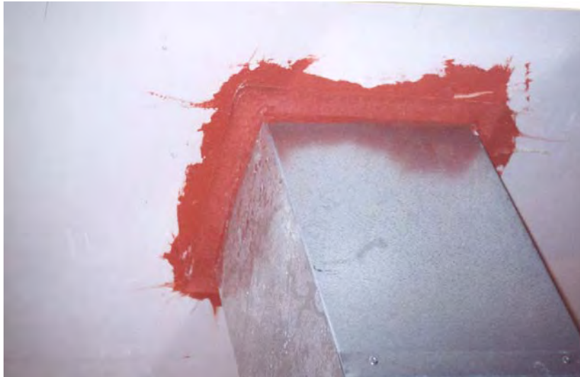
Figure 4: A Firestopping Sealant at a Through-Wall Penetration. While the primary focus of the sealant is to prevent fire and smoke migration to adjacent areas in the case of a fire, it has the secondary function of preventing everyday air flow, isolating possible pollutants and irritants in one room from another.
